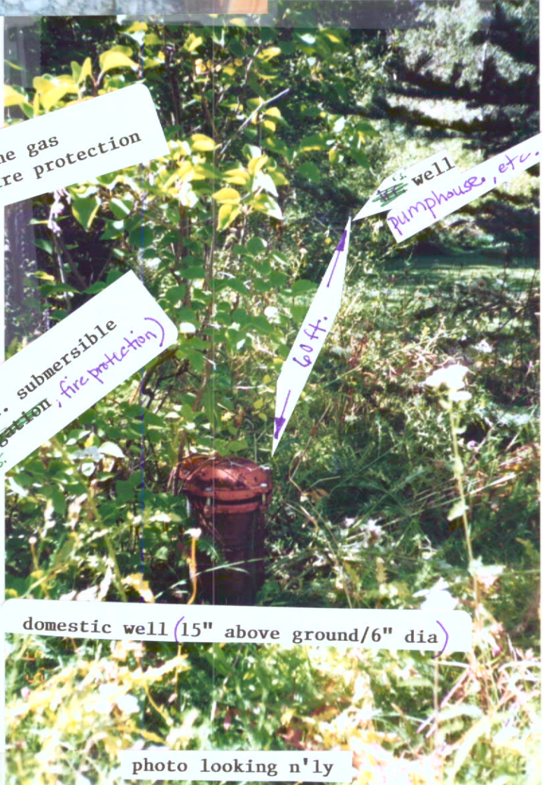
pipe supplies water to the pond and sprinklers
