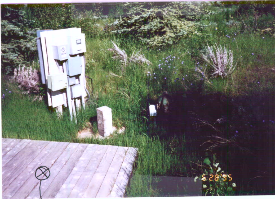
Piping System Cover
