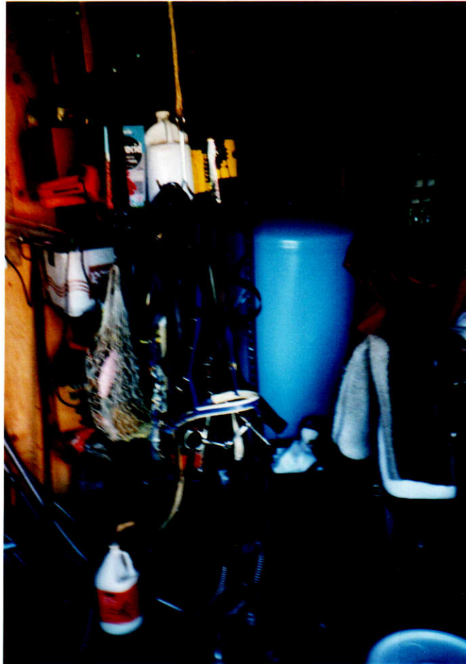
PRESSURE TANK IN SHED
