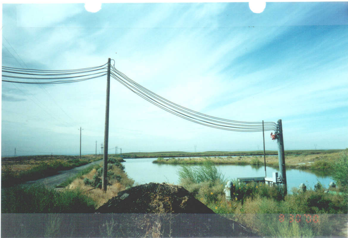
Well, Pond, Re-lift Pumps (Looking South)
