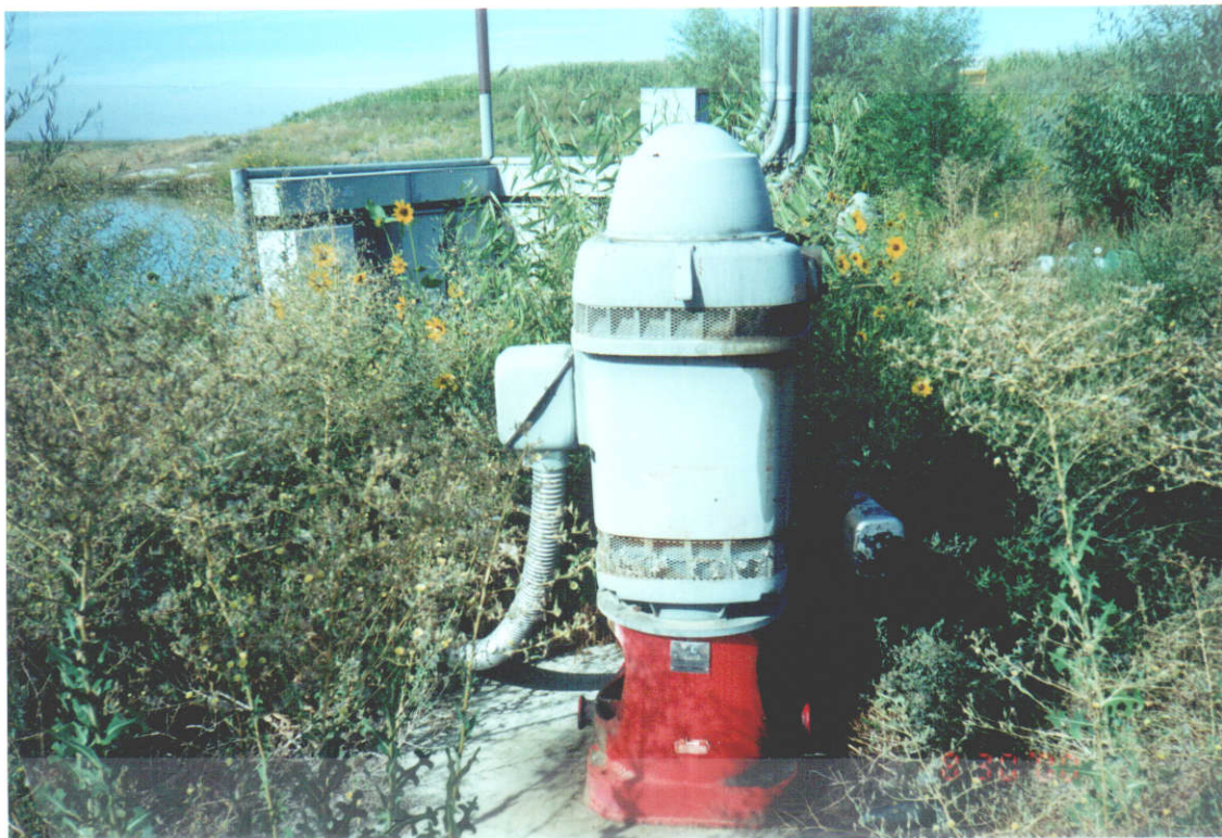
Closeup of Well (Looking West)
