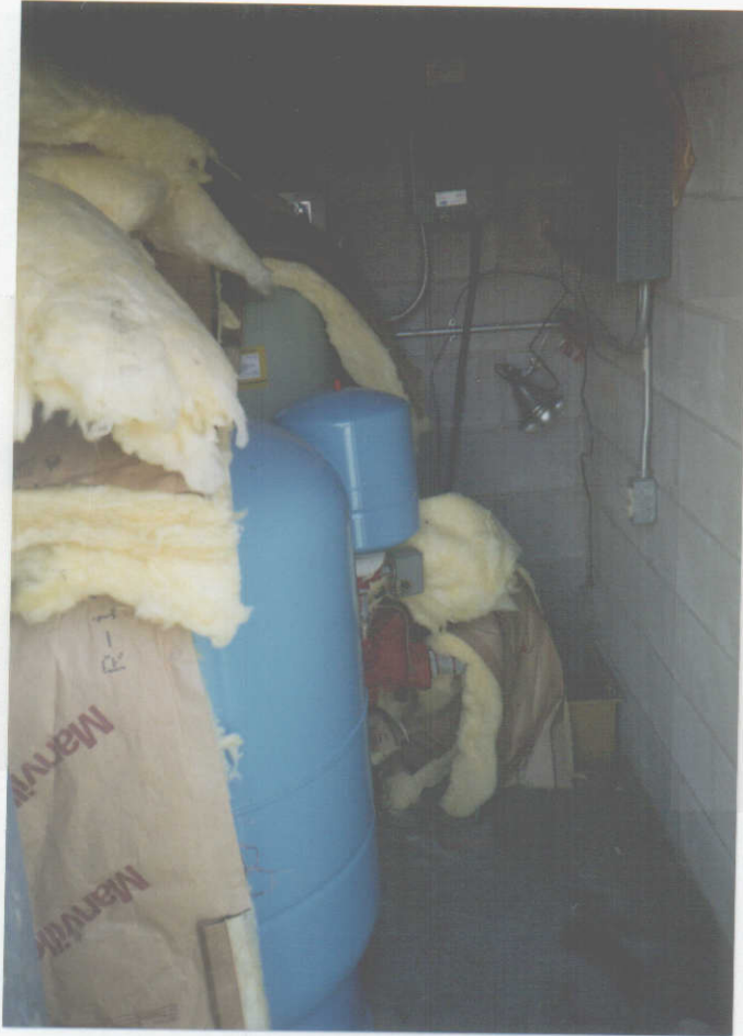
P/D - INSIDE PUMP HOUSE
