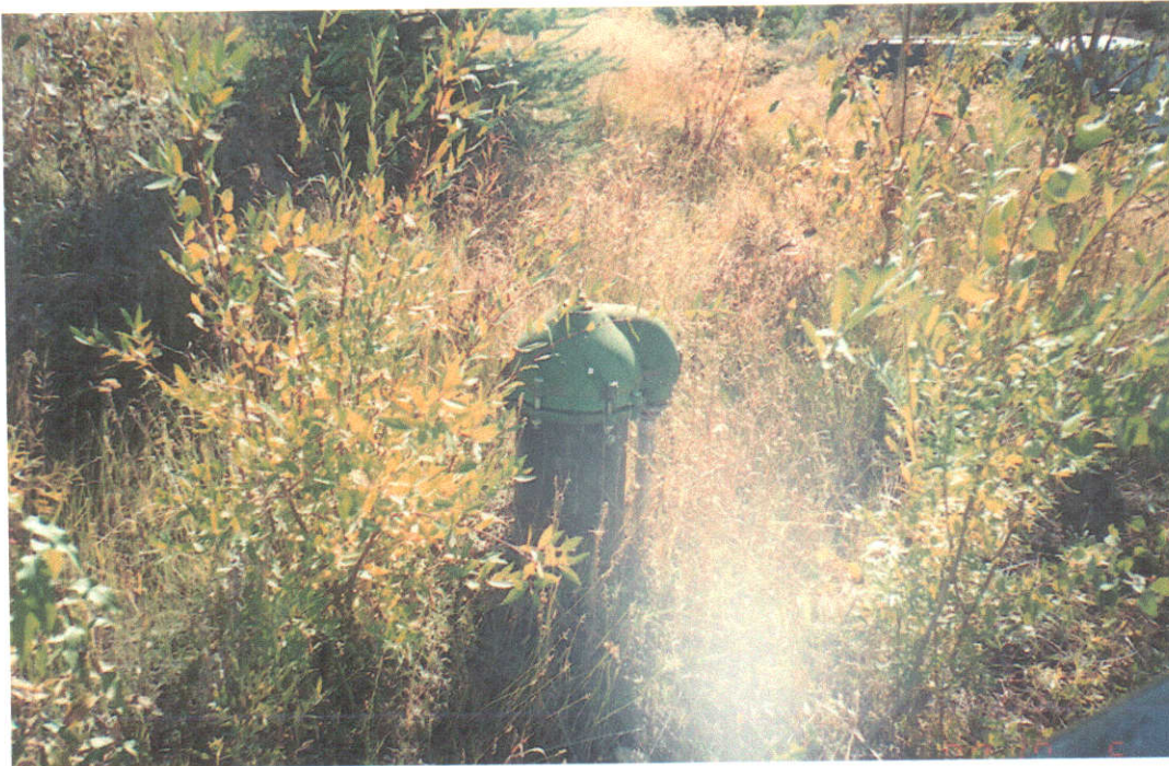
10" Dia Fire Protection Well - SE 1/4 NW 1/4 Section 1
