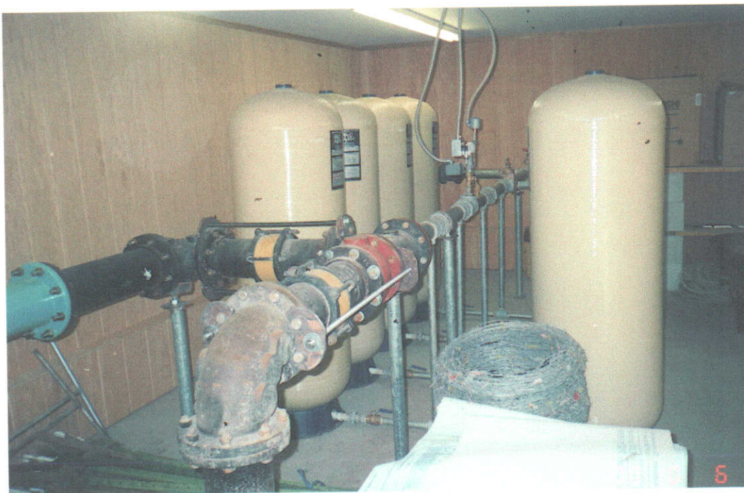
Inside well house showing pressure tanks, inlet lines, flow meter, & outlet line.
