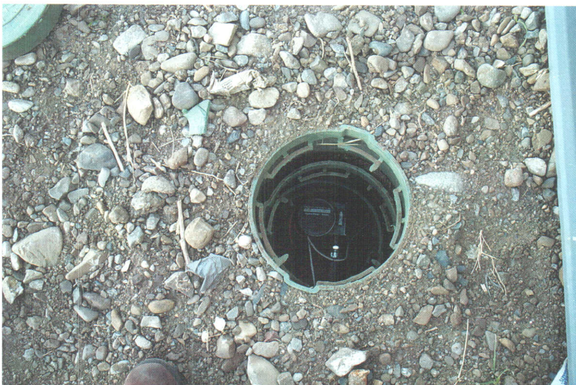
Flow Sensor In Mainline East of Well By J E Stanton 10-9-2002
