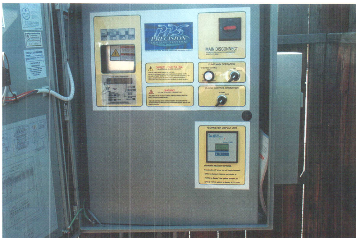
Closeup of Drive Control & Flow Meter Readout Inside Well Enclosure By J E Stanton 10-9-2002
