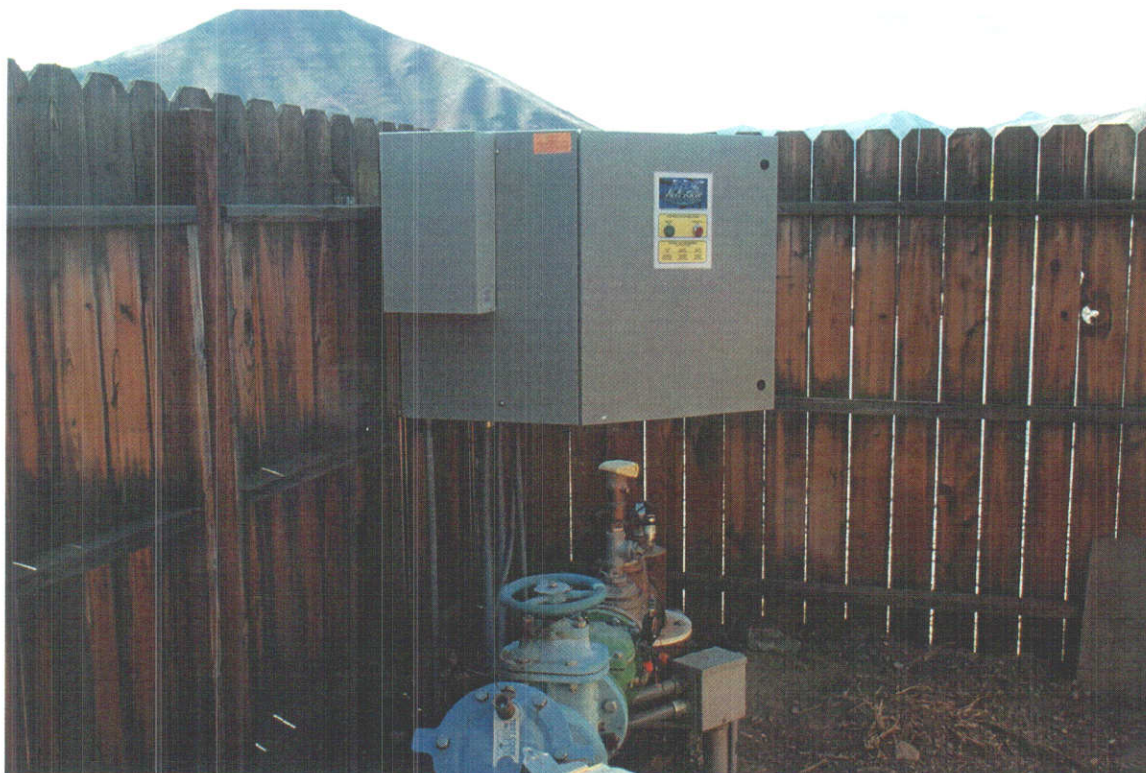
Irrigation Well, Control Box For Variable-Frequency Drive By J E Stanton 10-9-2002 Permit 37-8821
