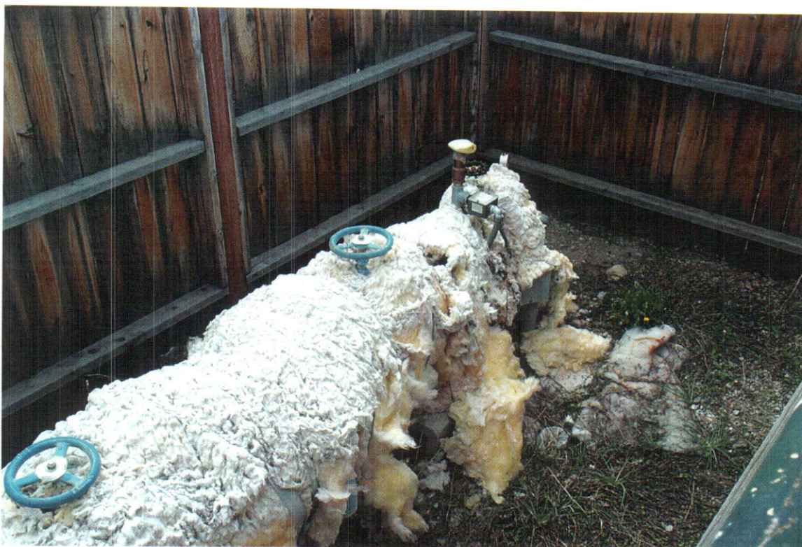
Well Head & Mainline With Insulation By J E Stanton 5-2-02 37-8821
