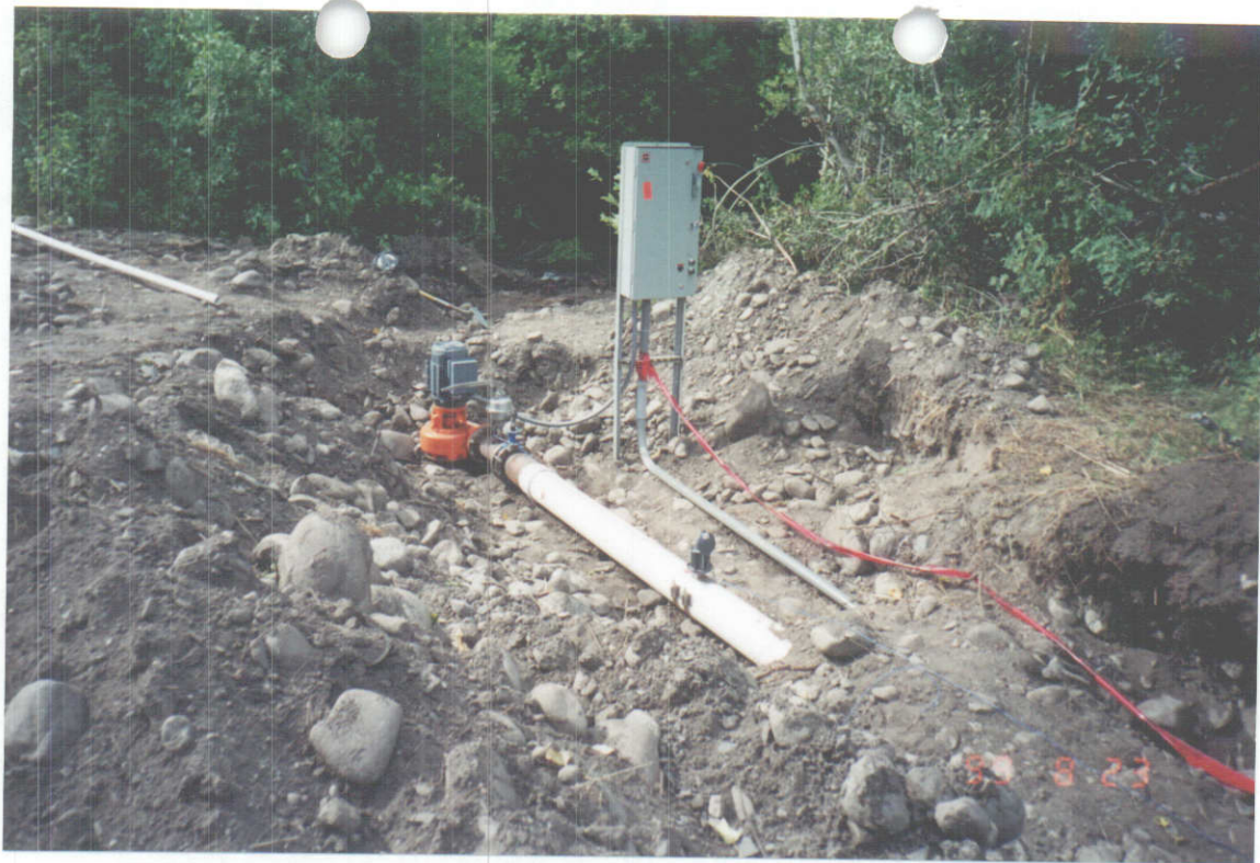
DIVERSION PUMP, VALVE, & 8" MCCROMETER FLOWMETER
