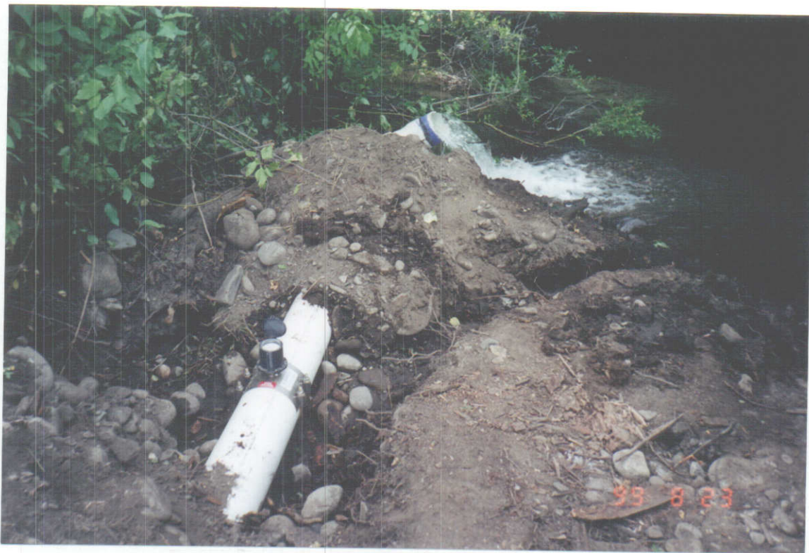
10" OUTLET PIPE & 10" MCCROMETER FLOWMETER
