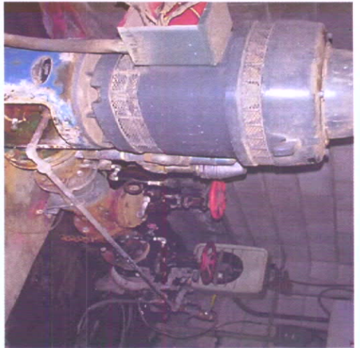
Outside Well 50hp pump
