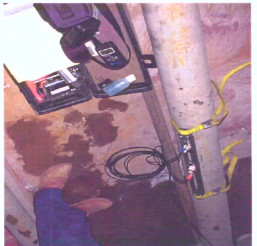
Inside well to right. Flow Measurement
