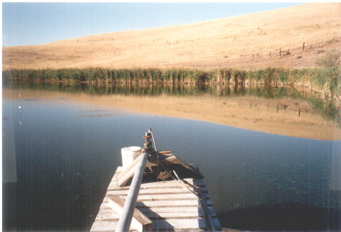
POND + PUMP FROM POND (PUMP STATION)
