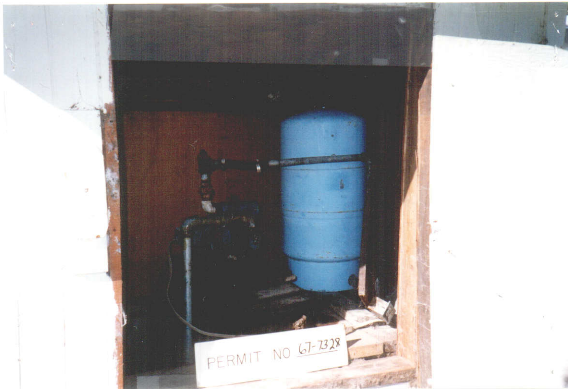
P.D. Well #2 Looking West
