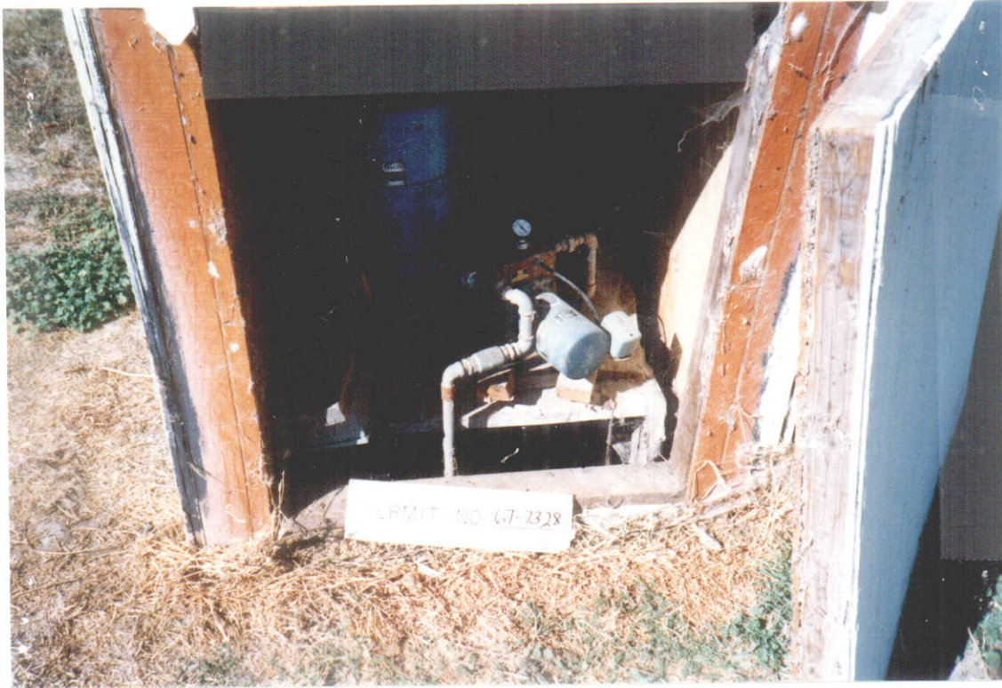
P.D. well #1 Looking West.
