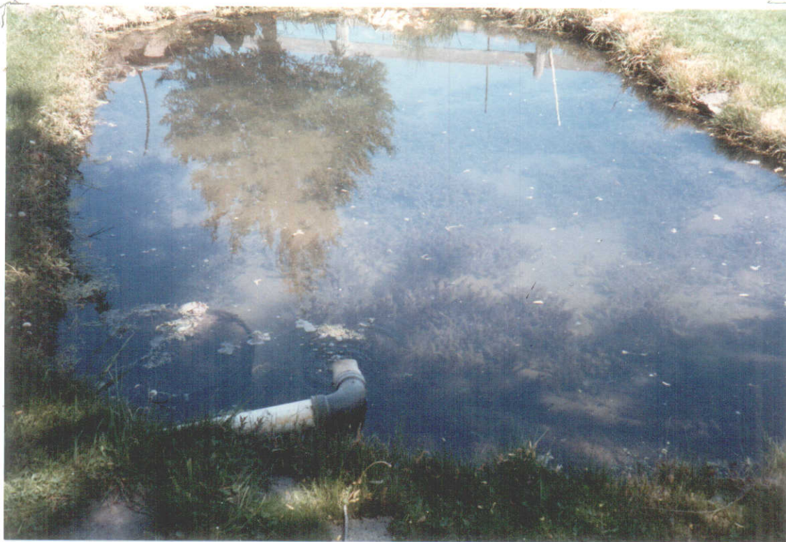
outlet pipe in pond #1 from holding basin
