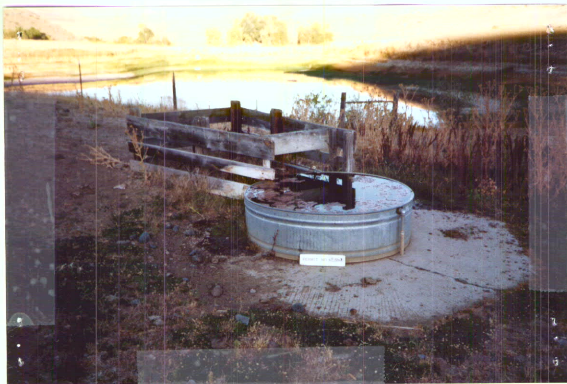
P.U. Well and stock trough. The pond in the background is not part of this system looking North west.
