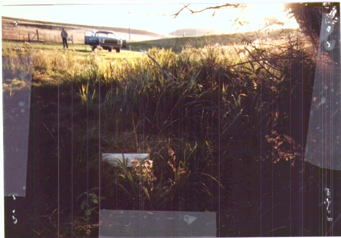
P.D. Looking Northeast The outlet pipe is overgrown and not visible.
