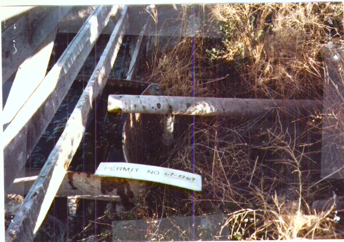
P.D pipe from spring. Looking North.
