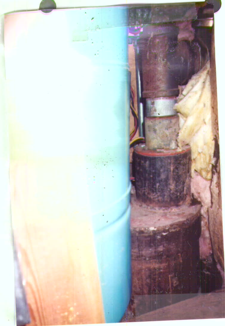
VIEW OF WELL CASING PRESSURE TANK. SYSTEM IS LOCATED NORTH OF THE P/U.
