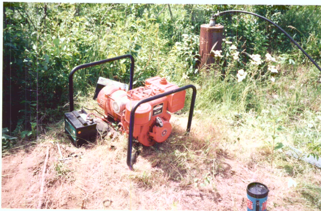
PHOTO TWO- Generator used for power to pump in well.
