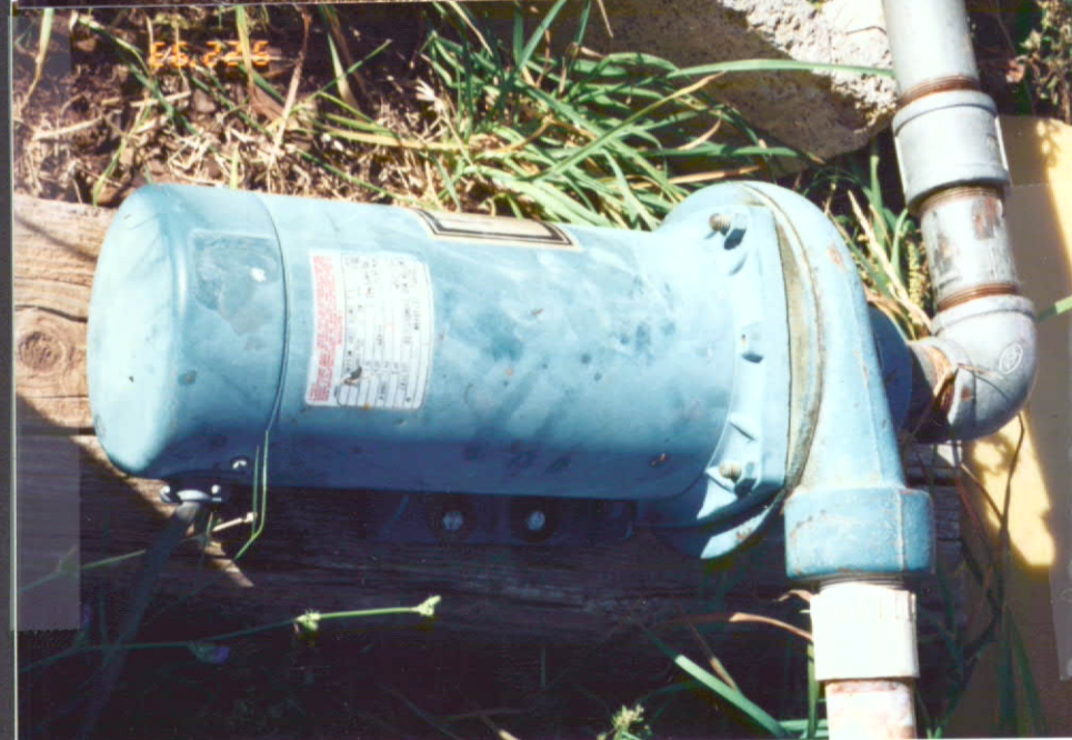
3. Centrifugal pump, 2 hp.
