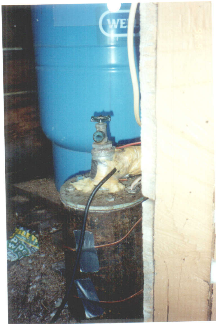
P/O a pressure tank
