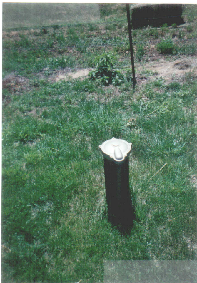
View of Well. Lines Go Underground to Pop-Ups in the Lawn to Spigots to Irrigate the Small Pasture.
