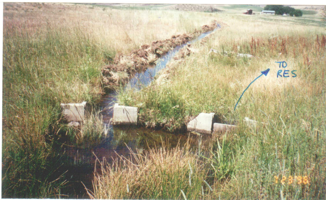
Split box in Sec 27. View to W. North ditch goes to Reservoir MICROFILMED
