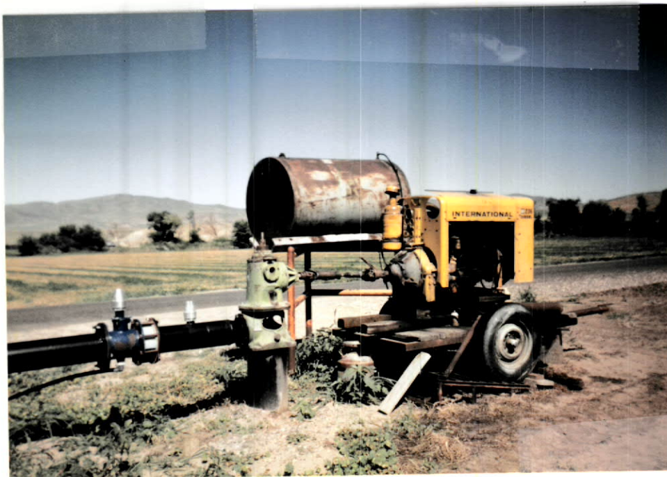
View of well, pump & PTO SYSTEM
