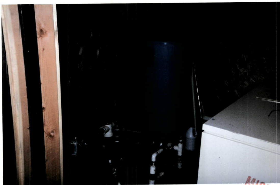
PHOTO TWO- well and pressure tank in well house
