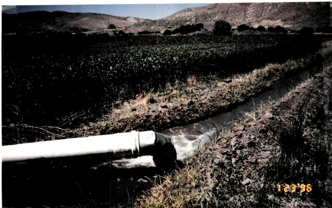
Discharge from pump and P/u field #1 (North) view to NW.
