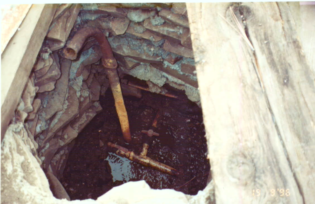
Junction box and drain to Creek. "T" to old home. (lines are leaking)
