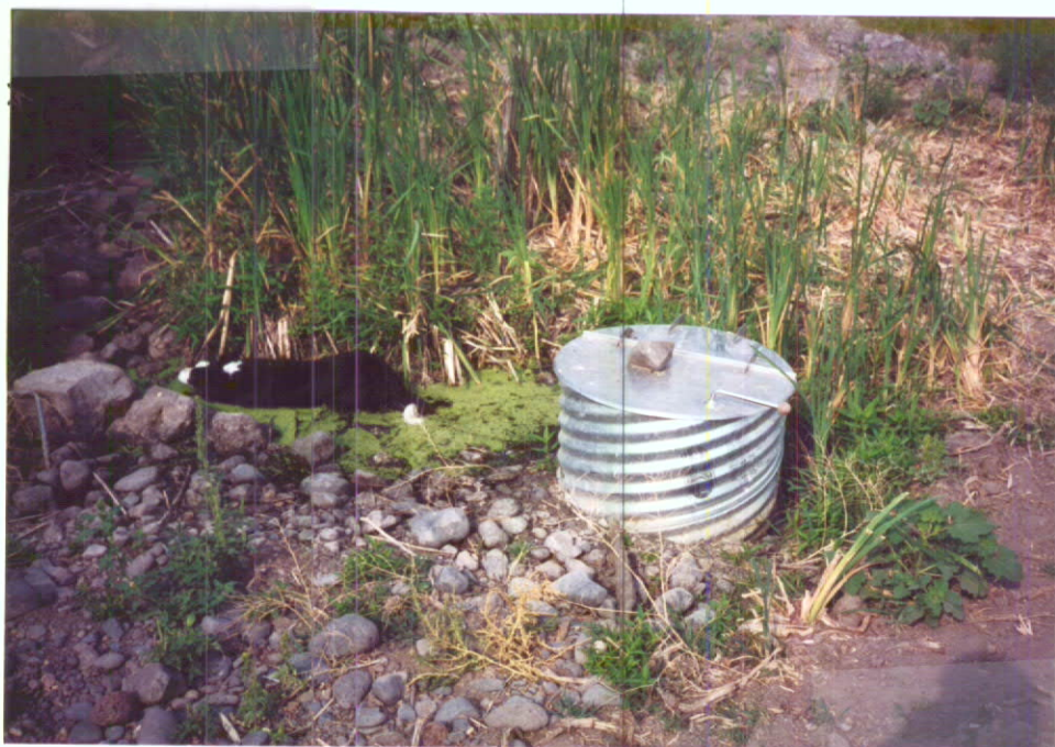
VIEW OF Collection box #2. The WATER SEEPS FROM A SMALL COLLECTION OF SPRINGS LOCATED AROUND THE box INTO A \frac{3}{4} " LINE THAT, THROUGH GRAVITY, FEEDS A STOCK TANK.
