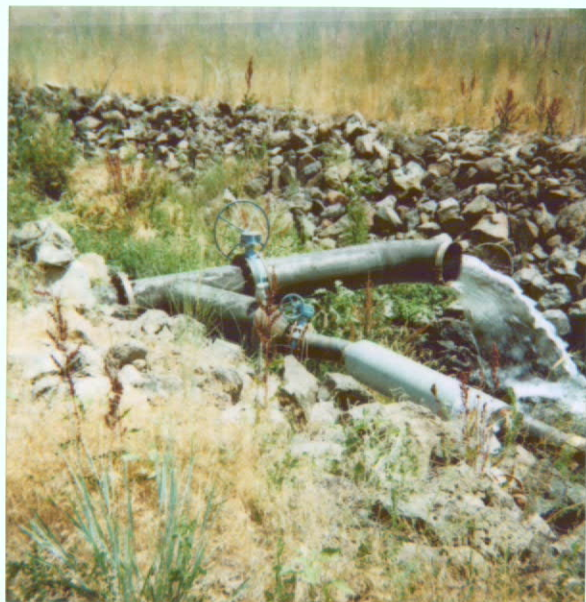
Irrigation Diversion from Reservoir
