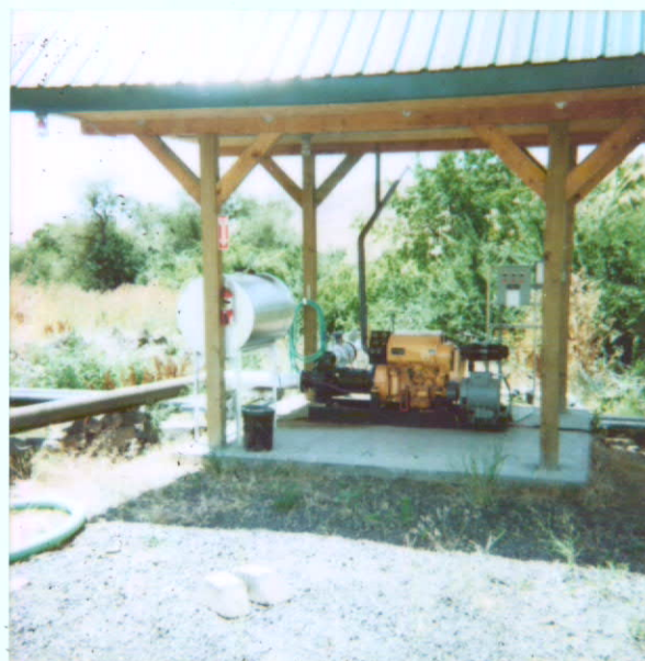
Diesel engine & Cornell pump from pipe at Res.
