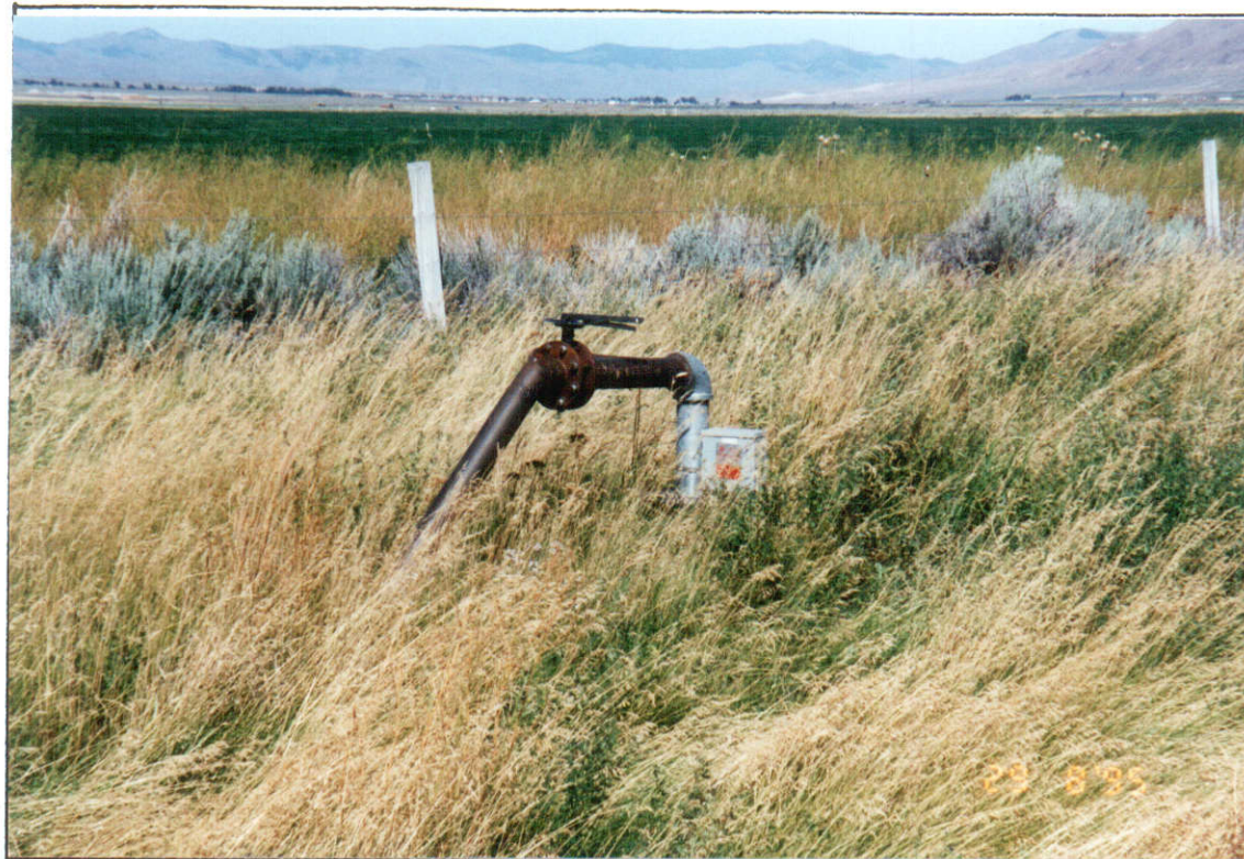
VIEW OF POINT OF DIVERSION SUBMERSIBLE 25 HP GOULD PUMP 16" WELL
