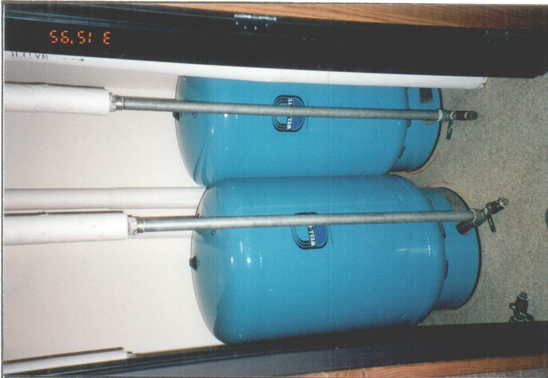
VIEW OF HEATING + COOLING SYSTEM + PRESSURE TANKS
