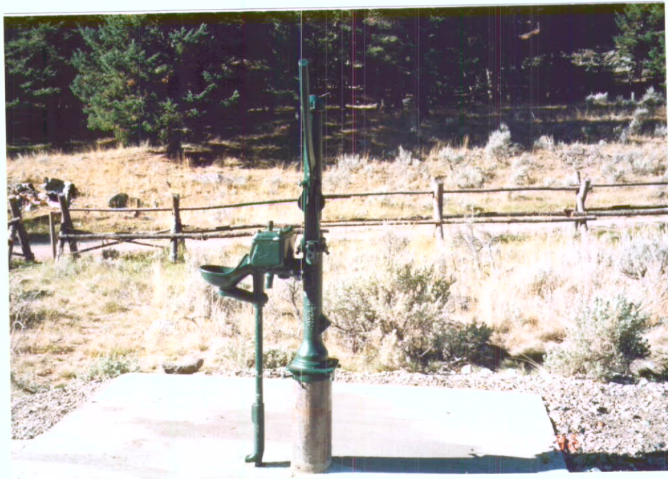
Well pump and surrounding jack fence to keep livestock out of well area.
