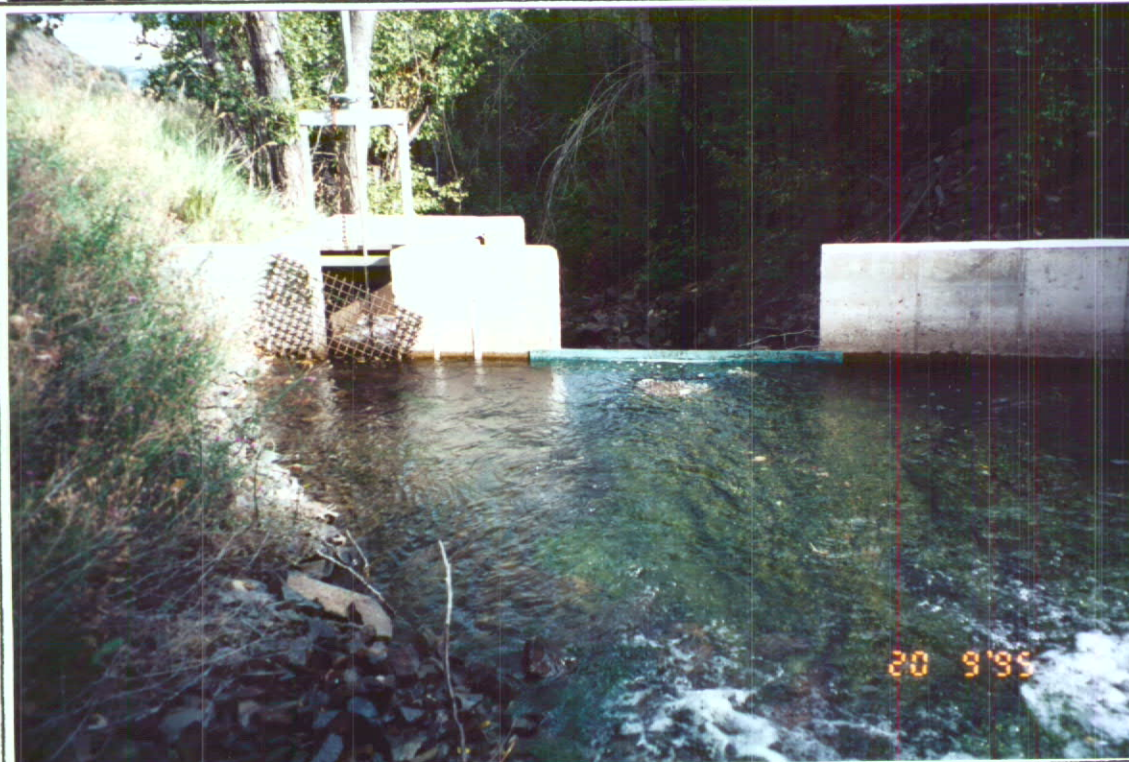
CITY OF SALMON MUNICIPAL WATER INTAKE ON LEFT.
