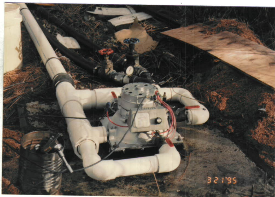
INTAKE TO POWER ALTERNATOR
