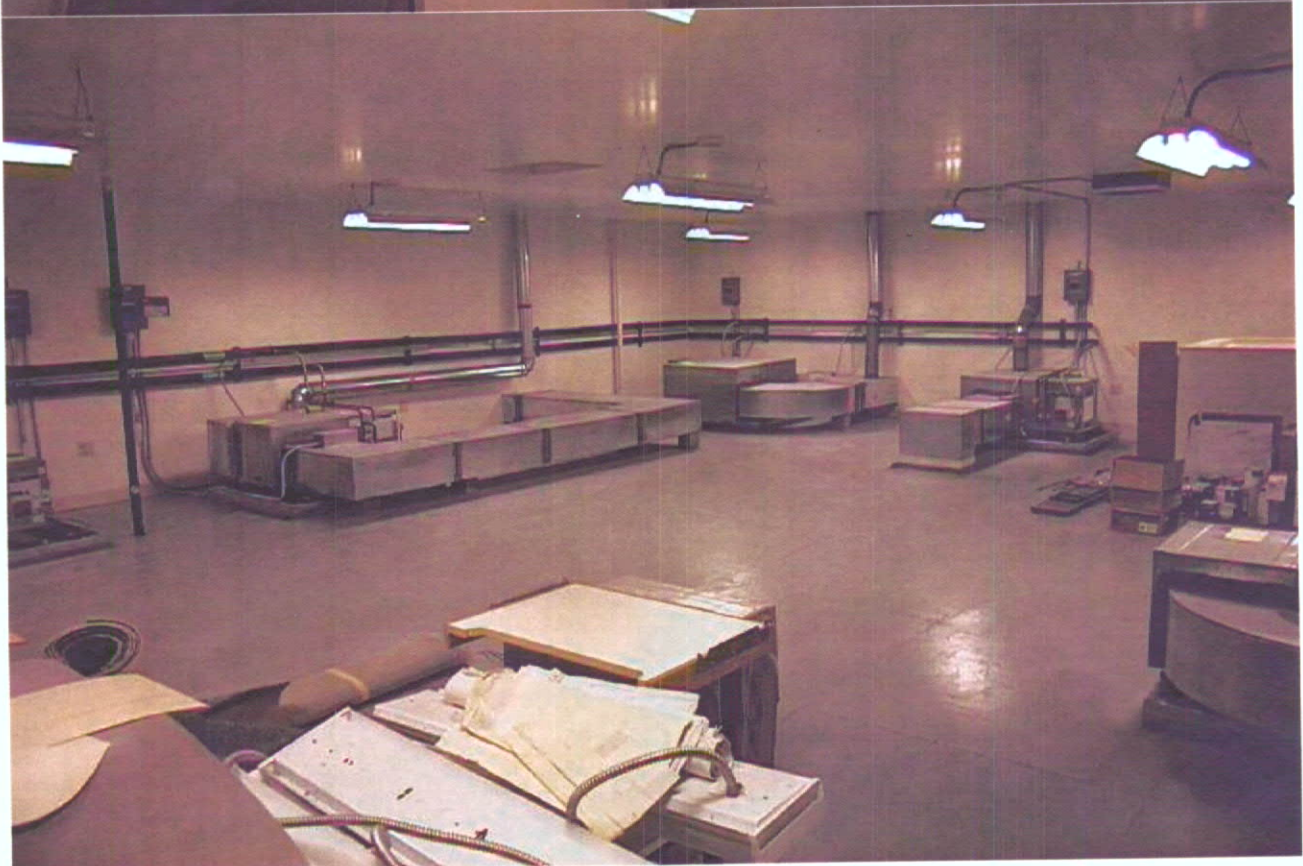
Six Heat Pumps for Heating & Cooling 75-07624
