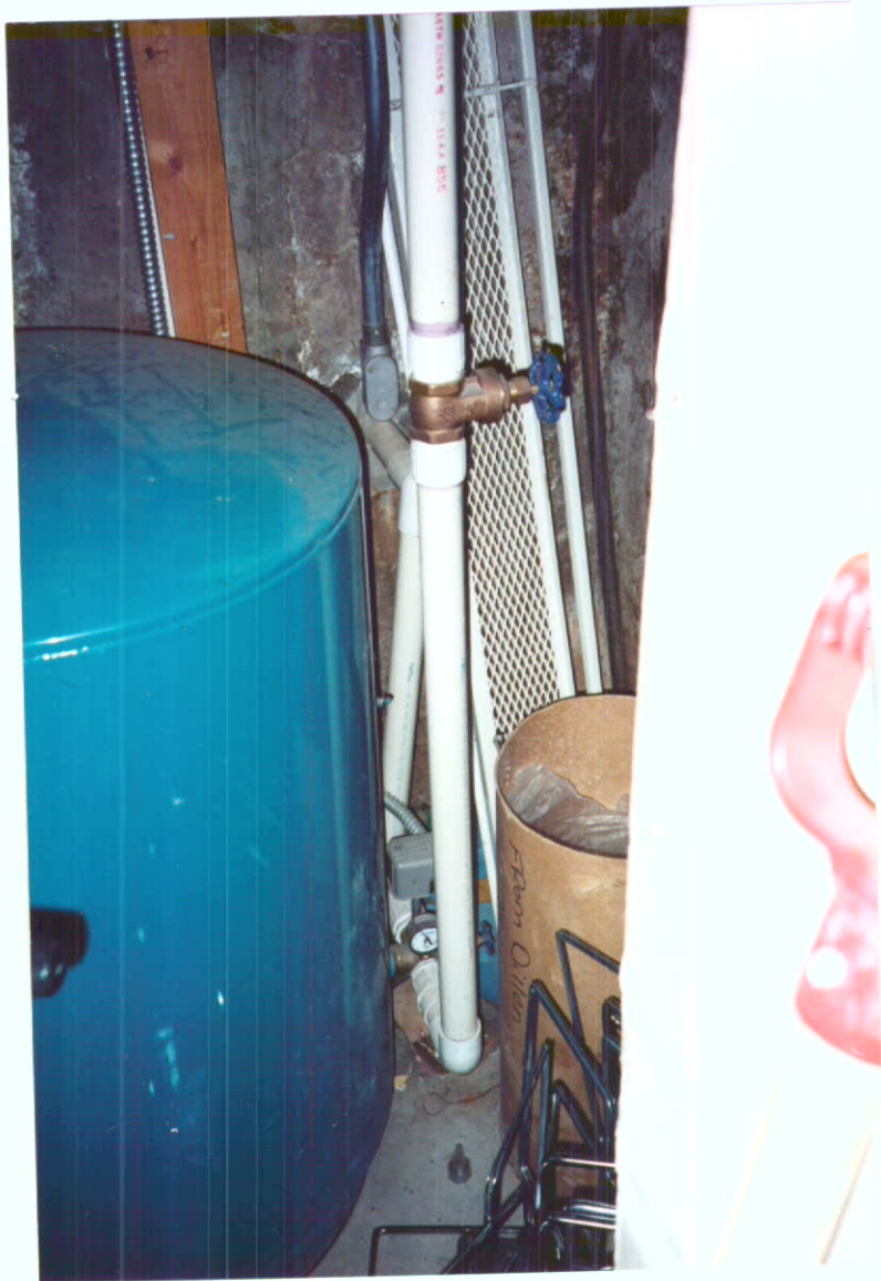
VIEW OF PRESSURE TANK, PRESSURE GAUGE AND GATE VALVES.
