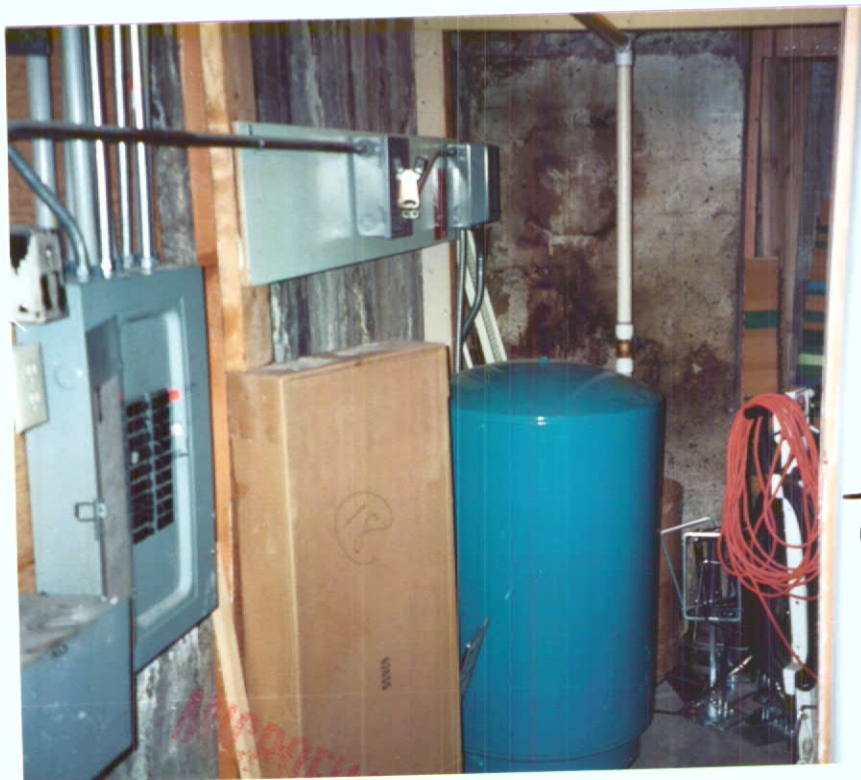
VIEW OF PRESSURE TANK IN BASEMENT
