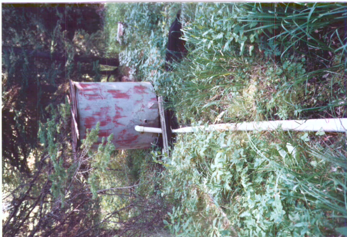
5' DIA. by 5' HIGH STORAGE TANK NEAR SPRING.
