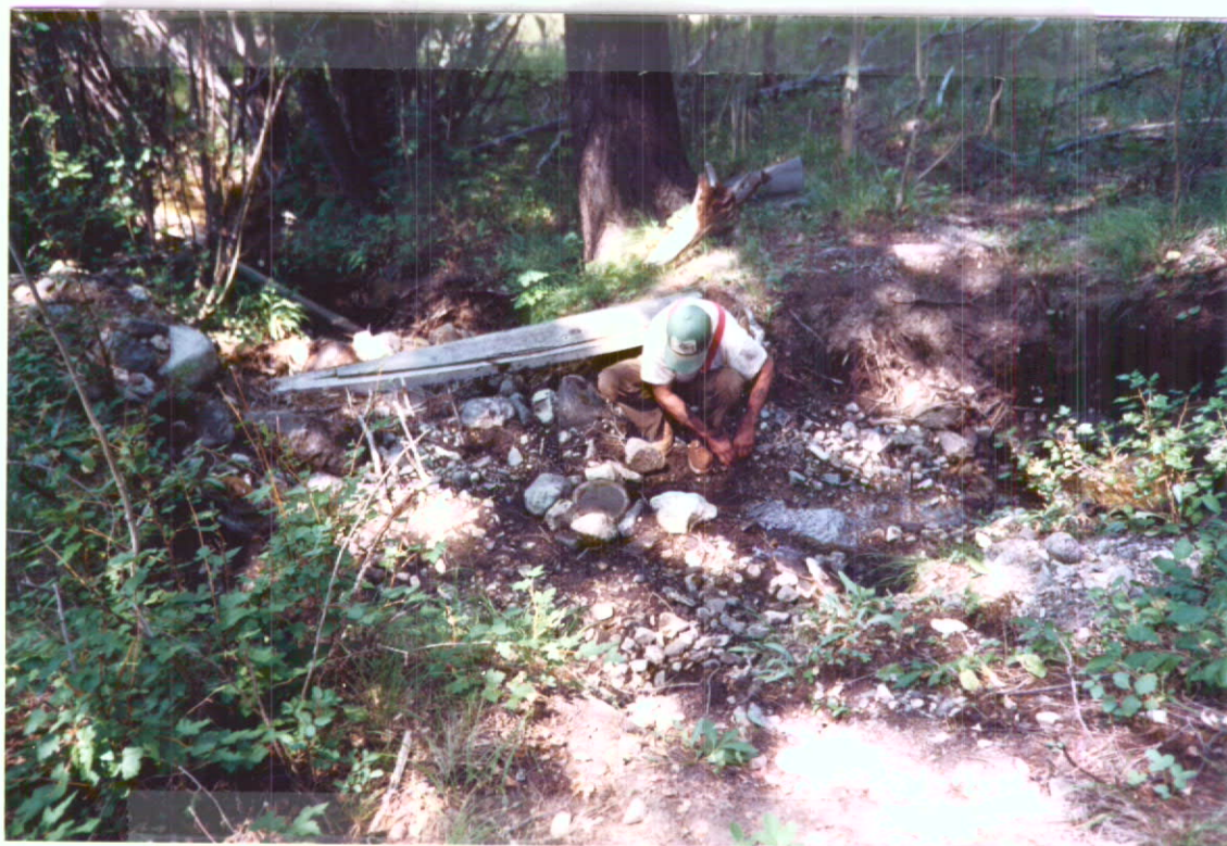
MR McAFEE CLEANING SCREEN INTAKE FOR PIPE TO HIS CABIN.
