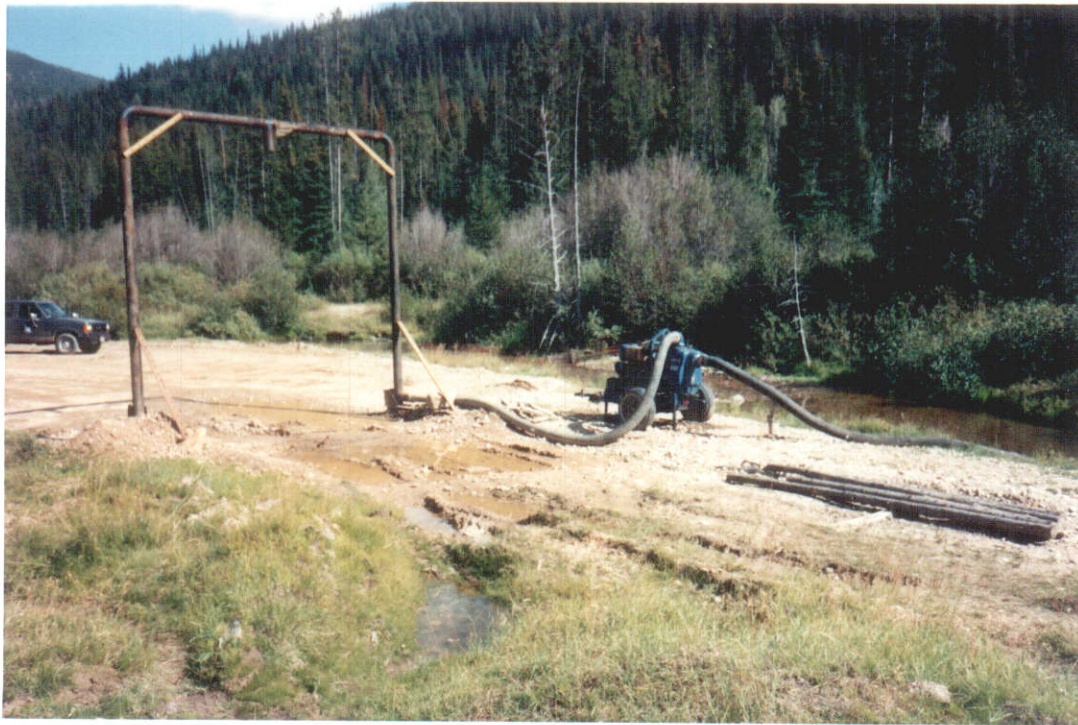
PHOTO FIVE NINE This is pump for 77-07071 (examined 8/18/89 by KRC). A similar pump system is used for 77-07293 (previous photo).
