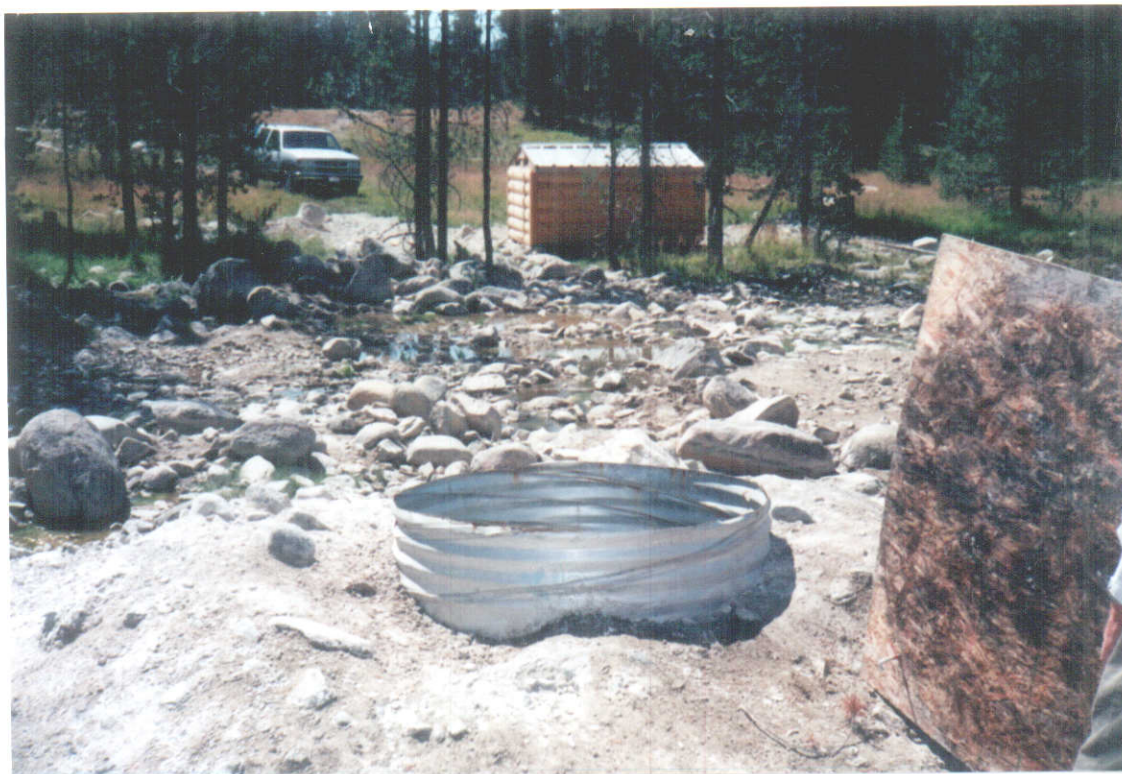
Hot Water Spring #3 & Pump House B.S.A. 8-19-00 77-07384
