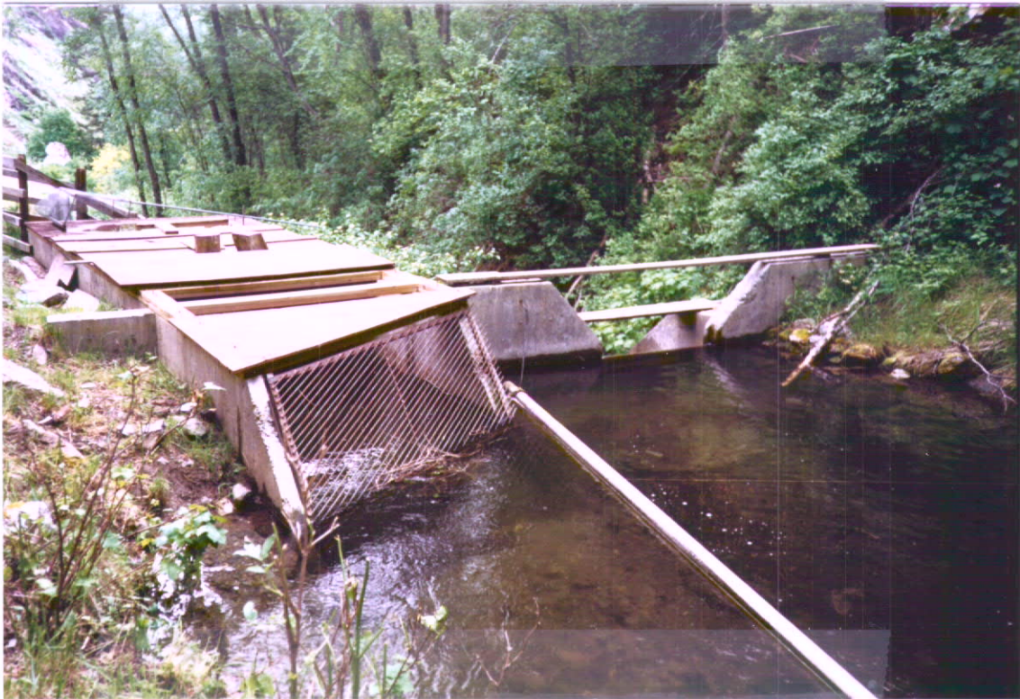
Diversion Into 14" Steel Penstock
