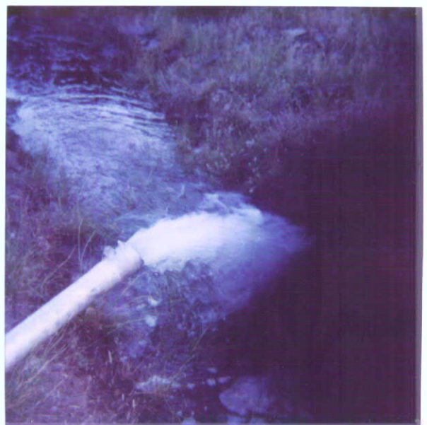
PUMP DISCHARGE & PORTABLE MAINLINE
