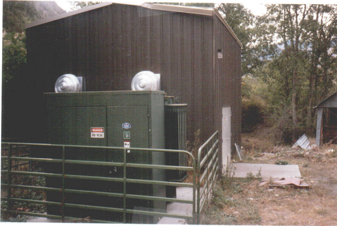
P/W. Powerhouse & Control Panel.
