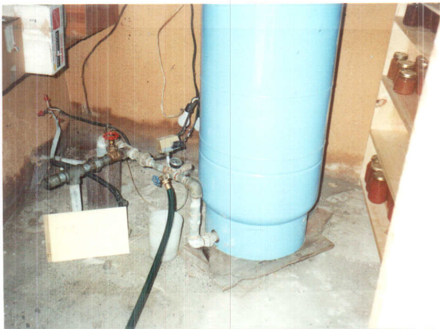
Picture of well & pump with pressure system looking south.
