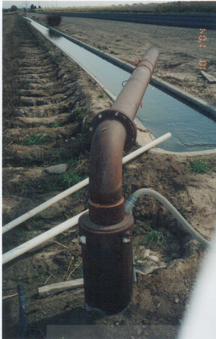
10" well, 10 HP submersible Pump open discharge located in the SWSWNE S30 T3N R2W
