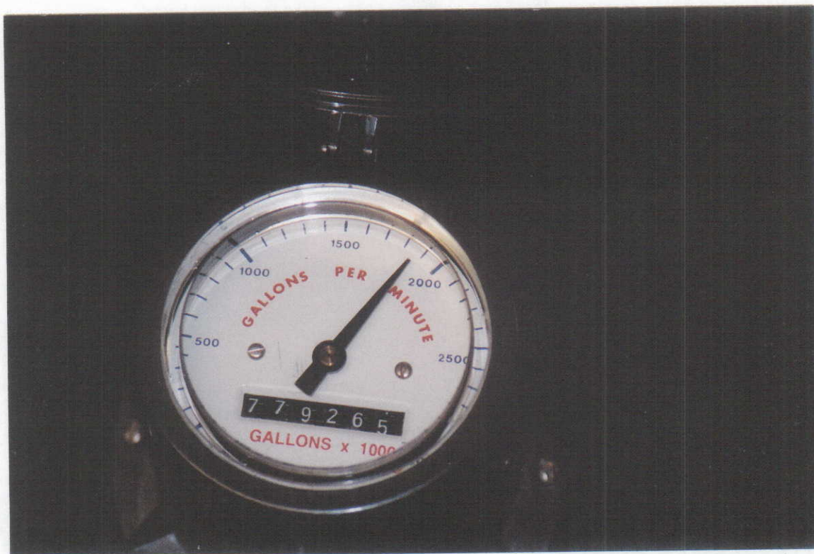
Figure 10. Photograph of the McCrometer totalizing flow-meter installed on the City of Meridian's #19 municipal water supply wellhead plumbing. Upper view is of the flow-meter prior to activating the well pump. The lower picture shows a discharge of about 1875 gpm after a few minutes of pumping. The discharge was held to a maximum of 1900 gpm for the 30-minute pumping test of this examination.
