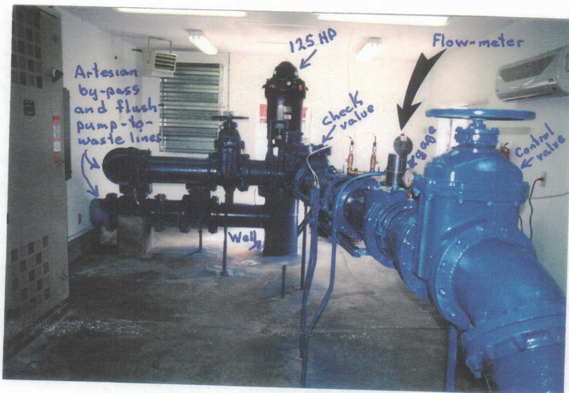
Figure 3. Photographs of the well head plumbing inside of the Meridian Well #19 pump house showing the configuration and specifications of the installed totalizing flow-meter.
