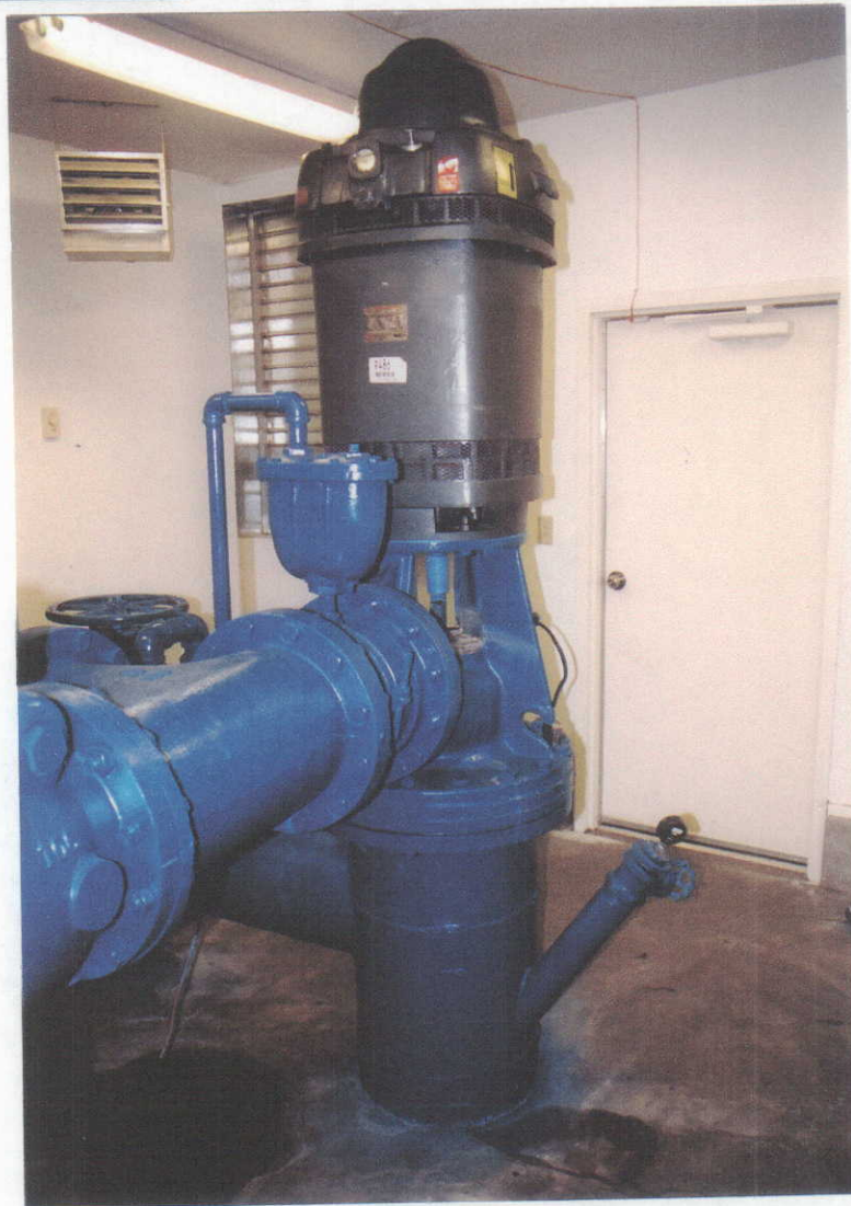
Figure 7. Photographs of the 125 HP drive motor for the line-shaft deep well turbine pump installed in the City of Meridian's 18-inch diameter #19 municipal water supply well. Upper view is a close up photo of the motor specification plate fastened to the motor.
