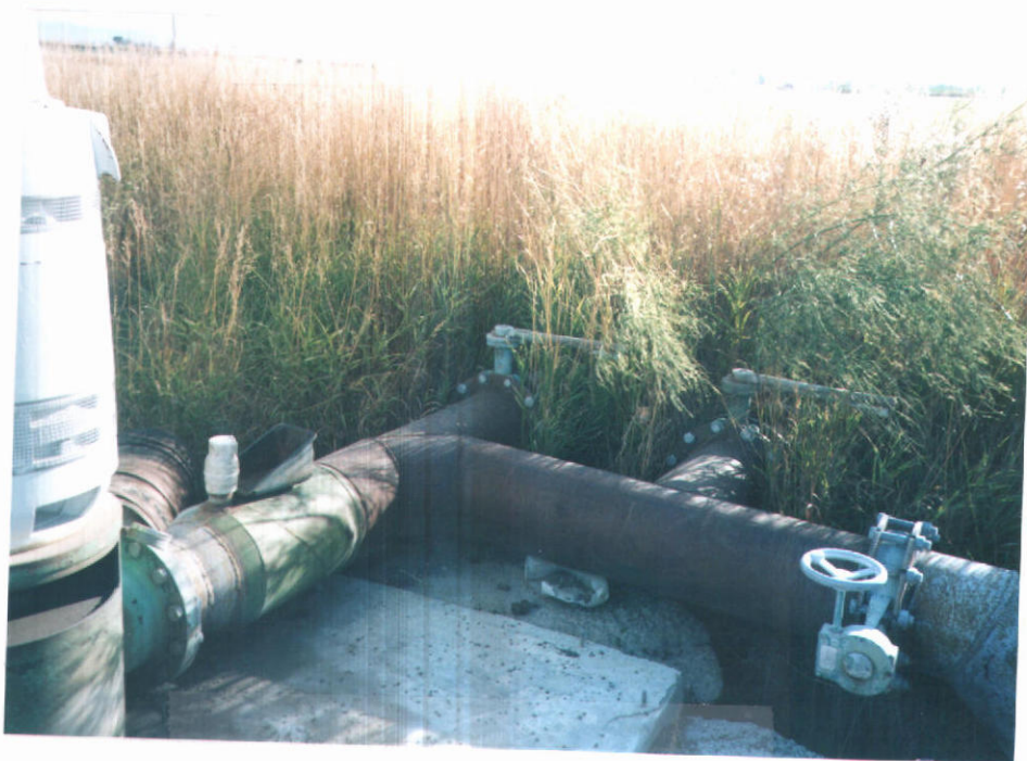
WELL/PUMP TO THREE WAY PIPELINE SYSTEM WITH GATE VALVES ON EACH PIPELINE.
