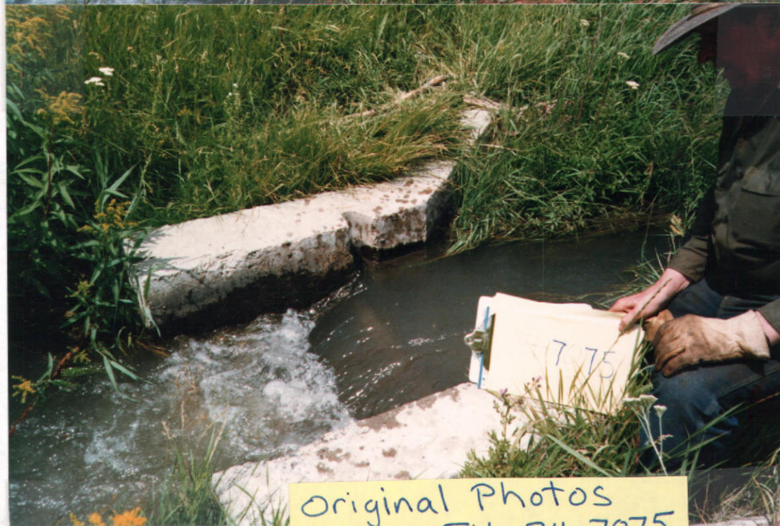
Submerged rectangular weir at Rediversion #2
