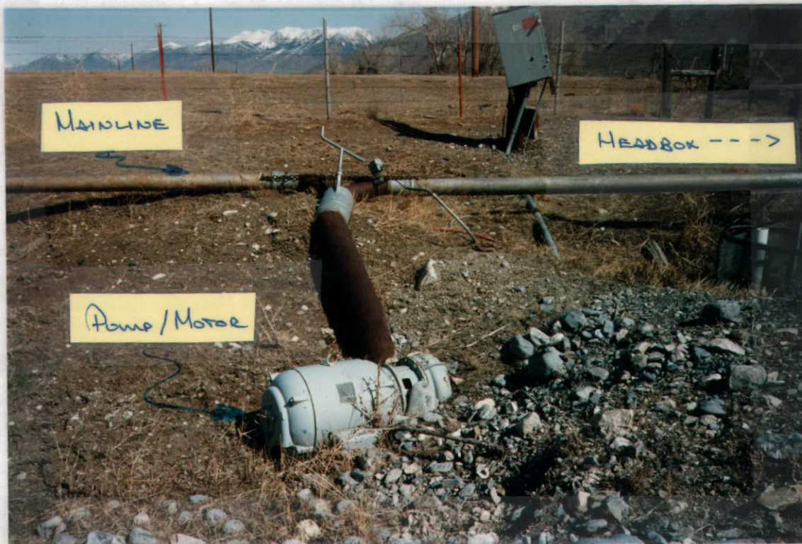
POINT OF REDIVERSION - PUMP, MOTOR, MAINLINE
