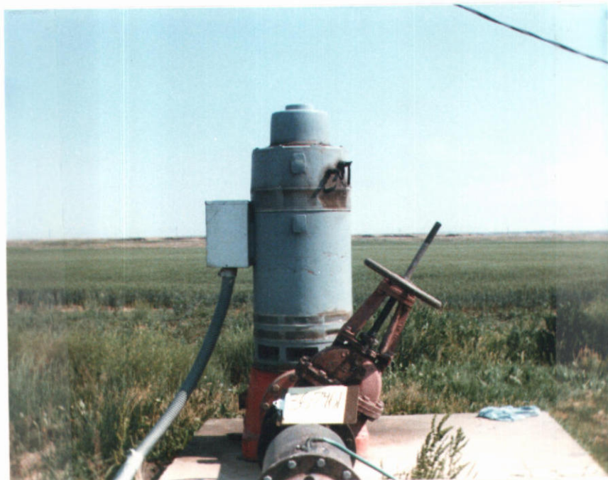
Point of diversion: Pump #2
