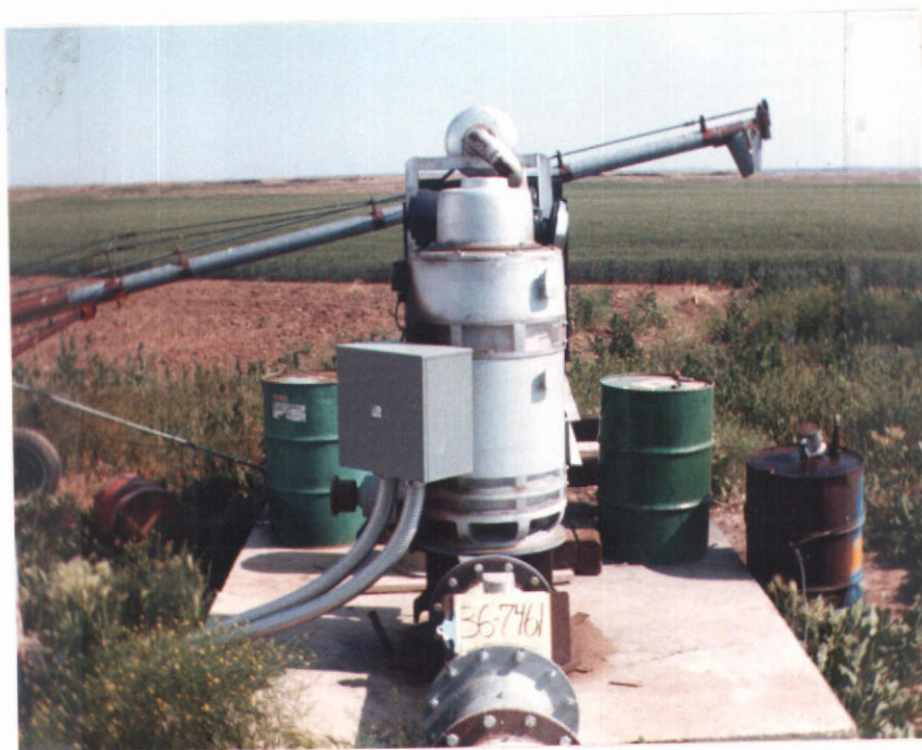
Point of diversion: pump #1
