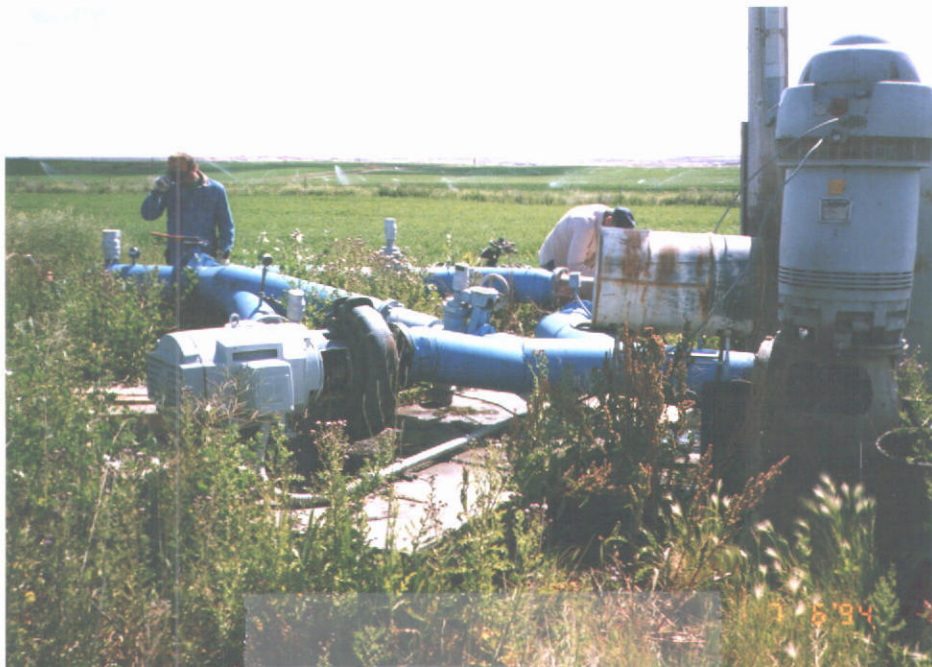
#2 P/O Pump Station #2
