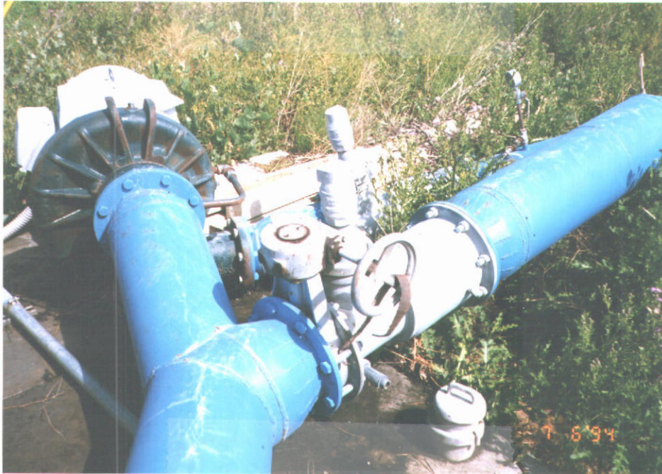
#3 West Booster Pump on Pump Station #2
