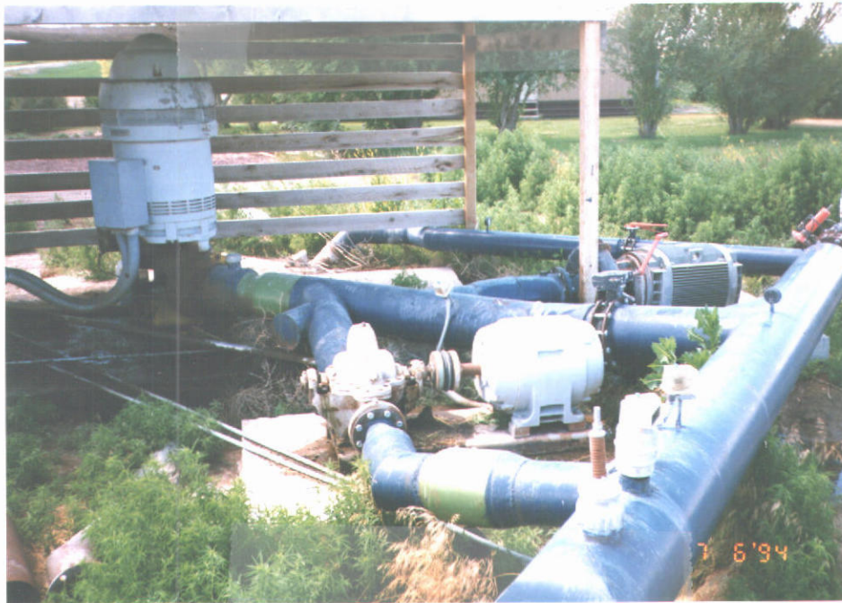
#1 P/O Pump Station #1
