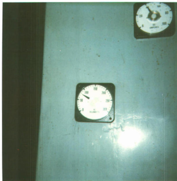
Power Meter - South Plant
